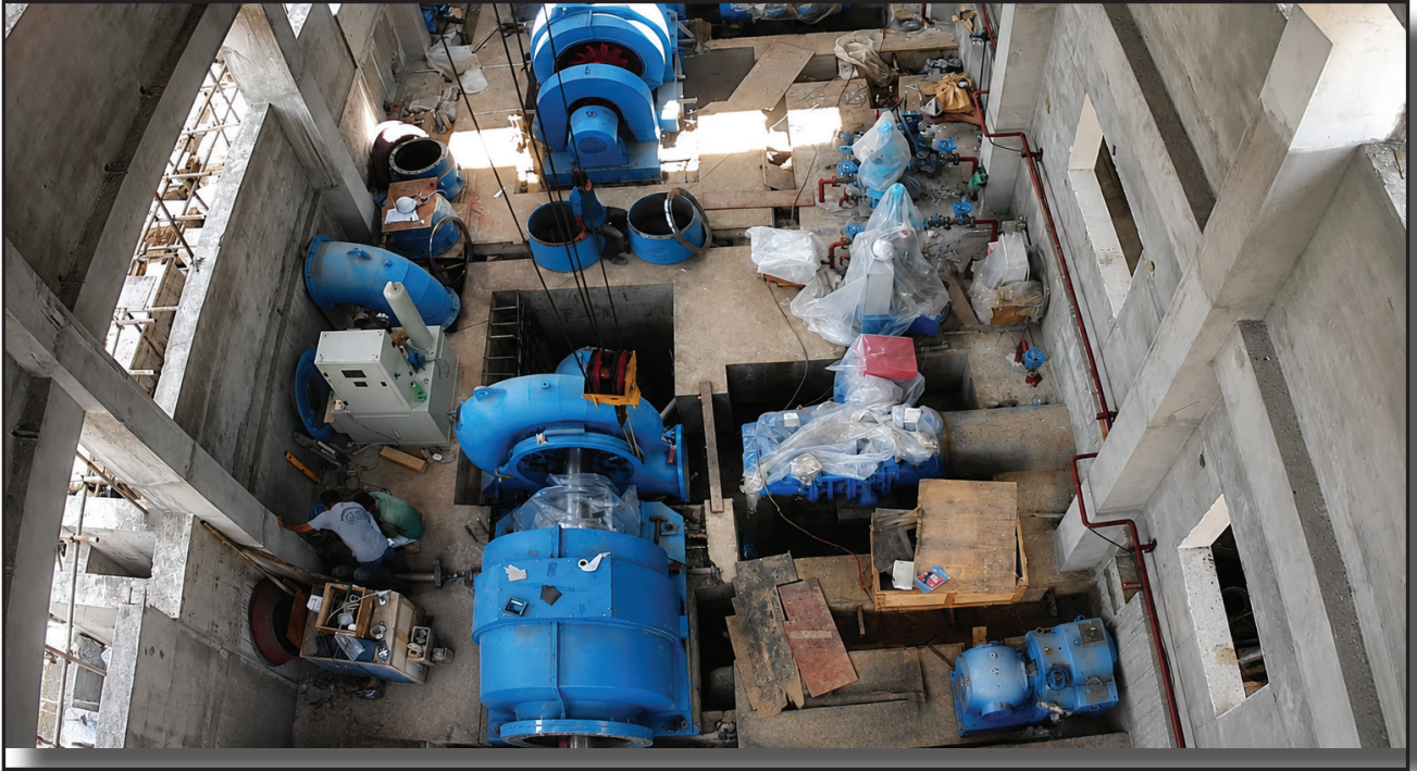
Cascade Machine Hall
